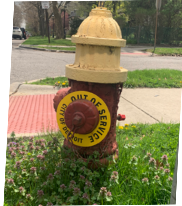
*** This picture shows the “collar” that DWSD that puts on hydrants that are out of service
